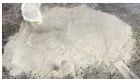
④ At first, give some water sufficiently into the hole, and then apply Boso 1 bann. Make even or smooth on the surface by a small hand shovel easily.
